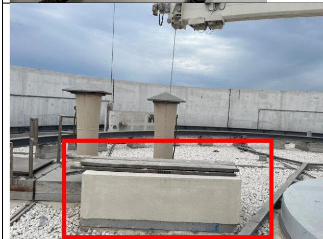
Rainwater catchment basin – is set to be refurbished to re-activate the existing infrastructure. Following completion of FJV Greywater system, the stormwater system will be integrated. Booster pumps (below) will pump greywater throughout the tower to feed apartment-level landscaping
